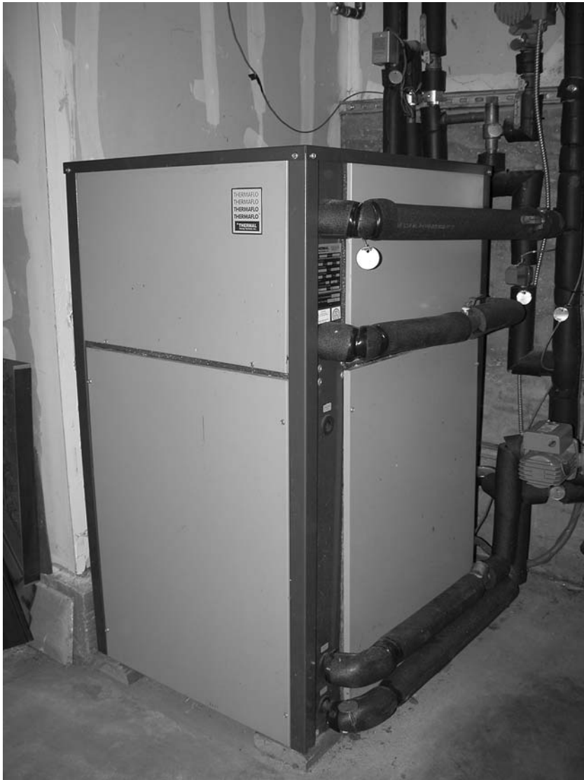
Figure 7.6 Photograph of Berkeley house geothermal heat pump.
