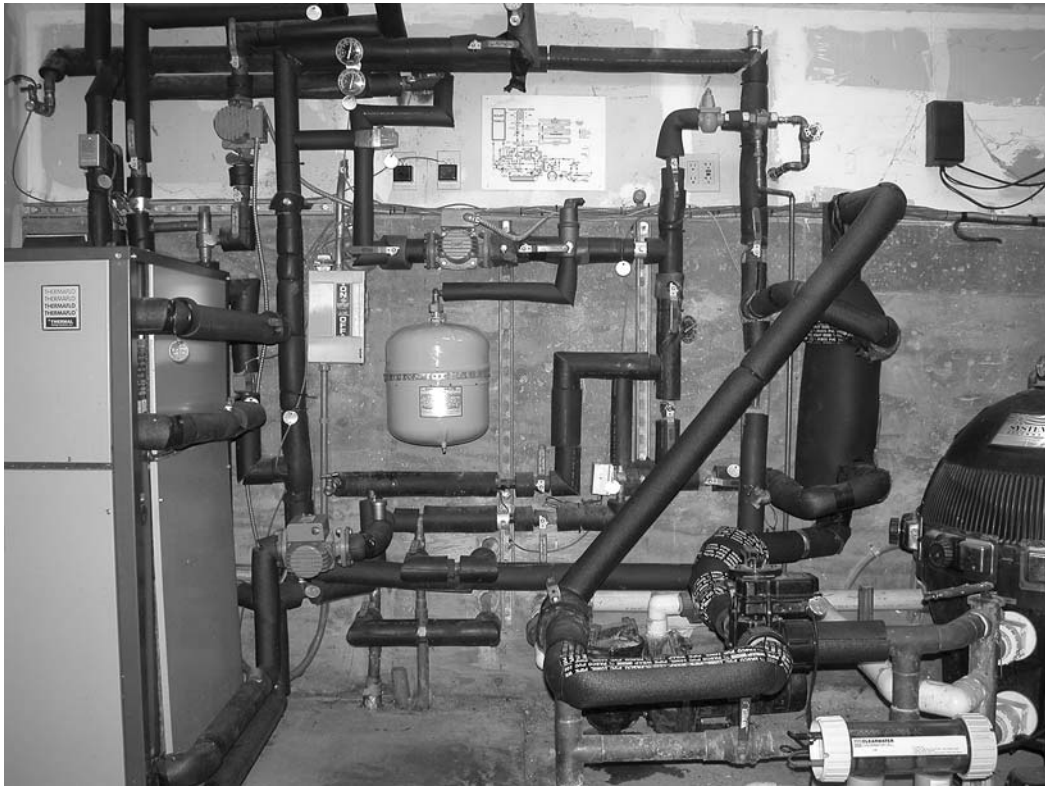
Figure 7.8 Photograph showing the solar piping/control system.
